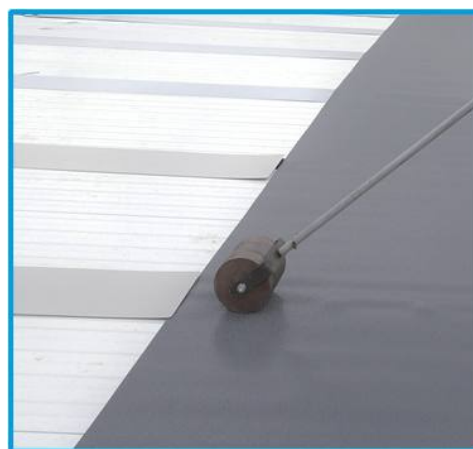
Rolling on the "Monarplan GF V (EM)" membranes using the "BMI InnoGrip pressure roller"
